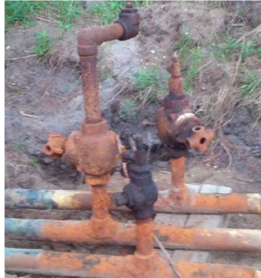
Figure 1 Valves Targeted for Repair
